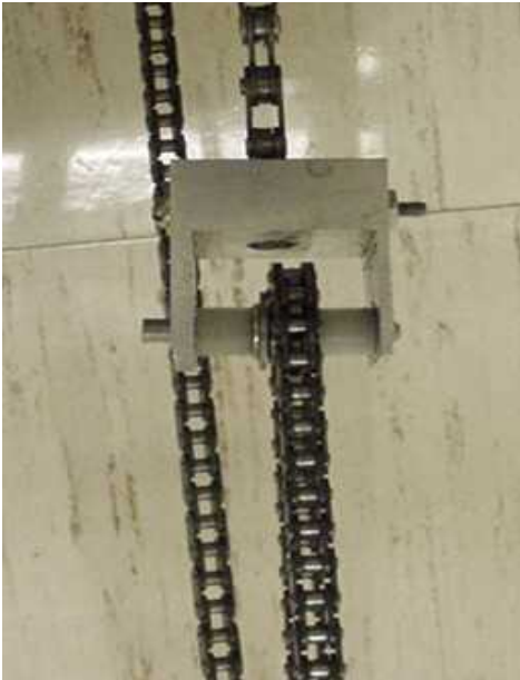
Picture 3: New Floating Pulley
